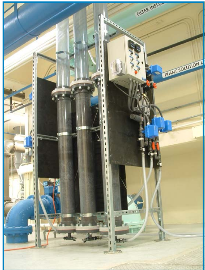
Automated Pilot Filters for Ozone/BAC Pilot
